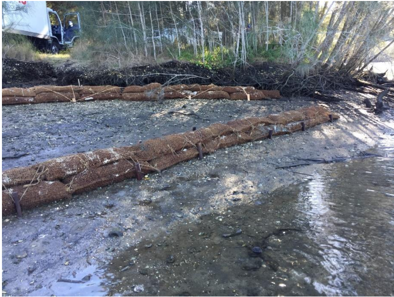
Photo 3.5. Structures installed at Sugarloaf Site.
