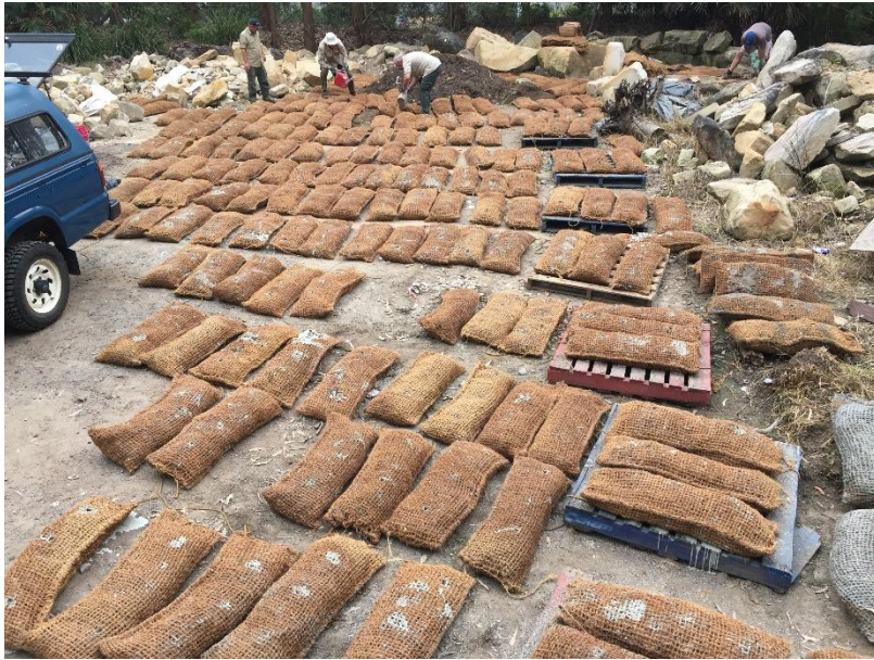
Photo 3.8. Photos of bags with concrete drizzle applied to bags of loose shell.
