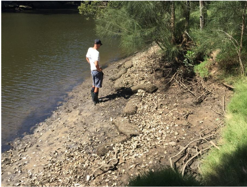
Photo 4.3. Photo of Judy's Elbow Site showing structure displacement - February 2019.
